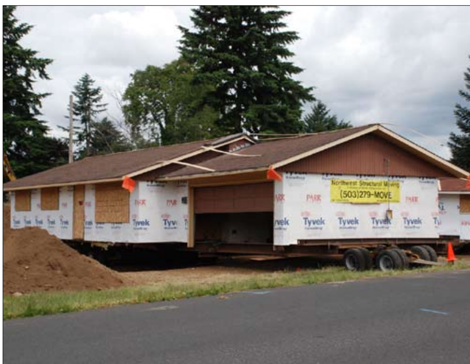
On The Move: A house is prepared to move from the construction site of Evergreen Public Schools' Health and BioScience Academy. The new high school will open in the fall of 2013.
